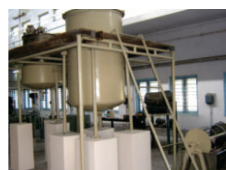
Fig. 19 Bleached lac Pilot plant
